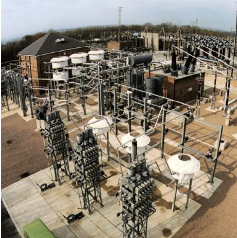
Photo 1.1: -75/+150 Mvar SVC National Grid Lovedean Substation, UK.
