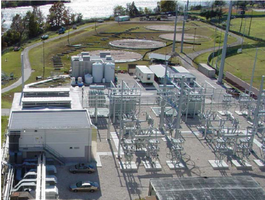
Photo 1.2: -100/100 Mvar 'Holly' STATCOM, Austin, Texas
