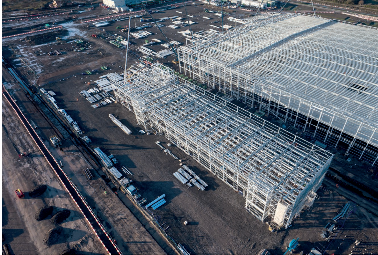
Agratas gigafactory, Bridgwater, Somerset, November 2025
