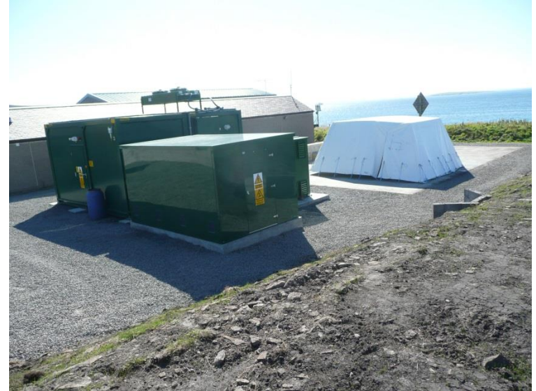
Transformer box at EMEC substation
