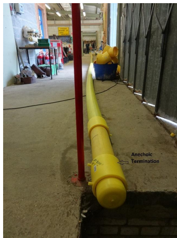
Figure 25. Photograph of anechoic termination in straight duct.
