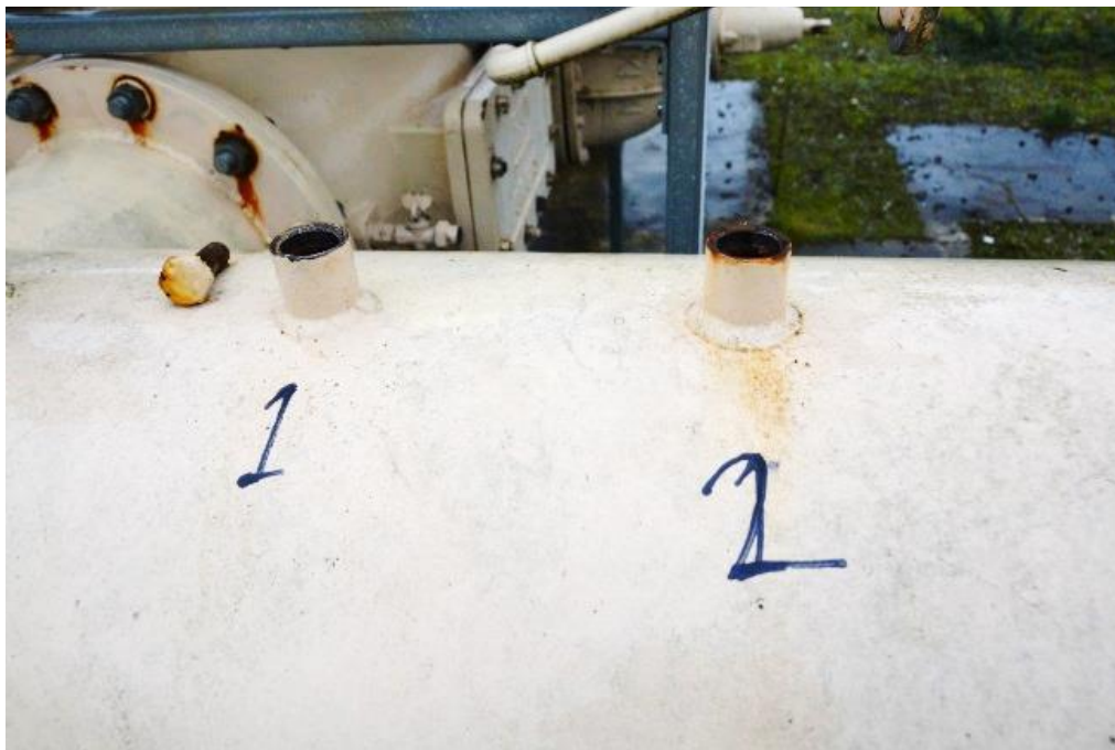
Figure 4. Microphones holders used to measure the sound pressure in a duct at test site in Northam
