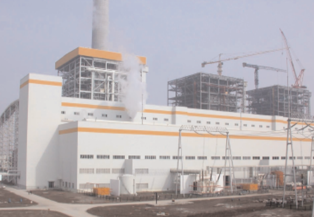
Figure 1. Changshu Power Station; 3 x 600 MW supercritical units under construction (courtesy of Mitsui Babcock)
