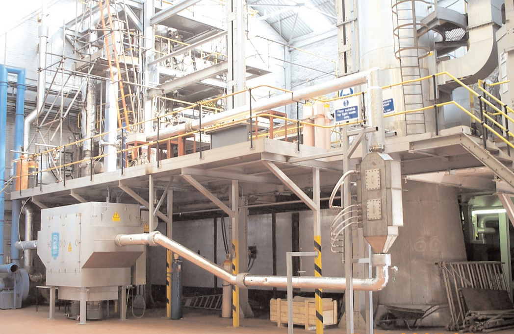
Figure 1. General View - NO x Reduction Test Facility (courtesy of Mitsui Babcock Energy Ltd)
