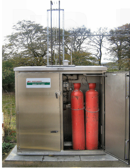
Figure 3. Hydrogen storage cabinet with vent pipes
