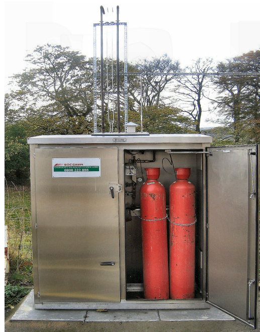
Figure 2. Hydrogen storage cabinet with vent pipes
