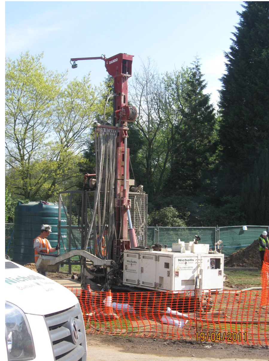
Figure 89 BTES Thermal Response Set Up
