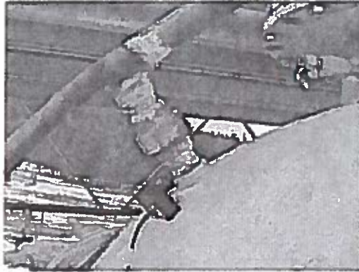
Photograph 6: AE sensor mounted for measurements on vent pipe 4
