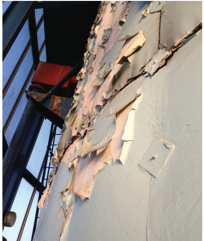
Figure 20. Superficial damage to the Accumulator's Plaster Coating
