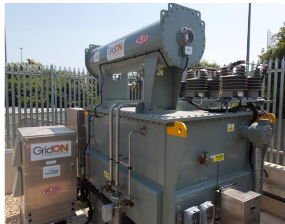
Figure 2 - PCFCL installed at Newhaven substation
