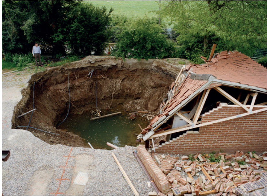
Figure 12. The impact of the collapse of karstic ground — collapse of four garages into a subsidence hollow caused by the dissolution of gypsum at Ripon, North Yorkshire in 1997. (Reproduced with the permission of the British Geological Survey © NERC. All rights reserved.)
