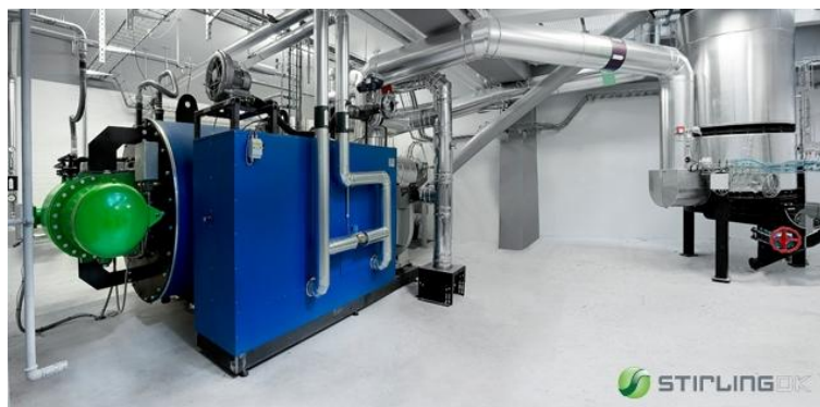
Figure 31-6 Updraft gasifier plant at the Technical University of Denmark (DTU). 35 kW Stirling engine on the left in green, combustion chamber in the centre in blue, and gasifier on the right (Stirling DK, 2011)
