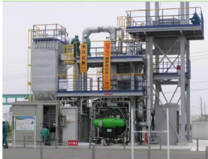
Figure 31-5 Wood chip furnace system with 5 Stirling engines (Stirling DK, 2010)
