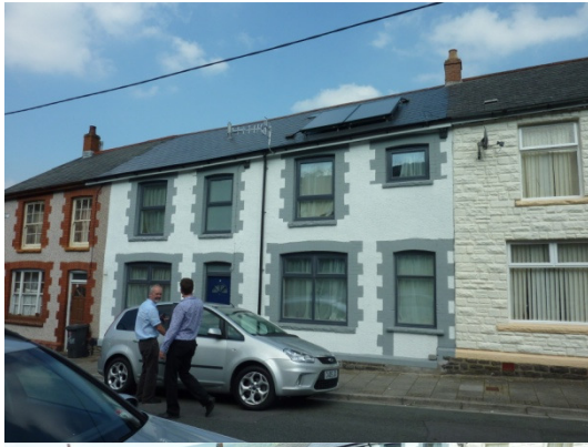
A newly completed retrofit property - solar panels on the roof are considered as a novelty in Wales. This property has been merged from two adjacent mid-terrace houses. The rightmost window has been converted from a front door into a window.
