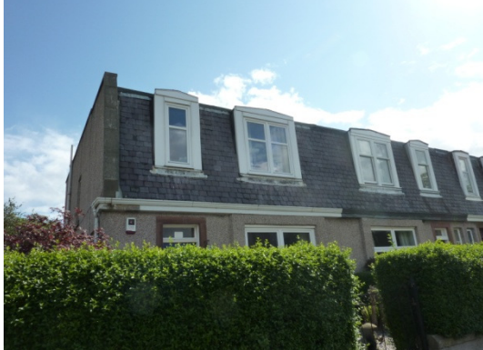
Mansard roof on a row of terraced houses. EWI would only tackle half of the problem in this case...
