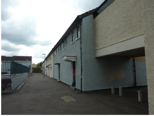
1950s terraced housing, presumably cavity wall housing with render finish. Potentially ideal for an EWI solution, as the internal spaces may be too small for an IWI installation.
