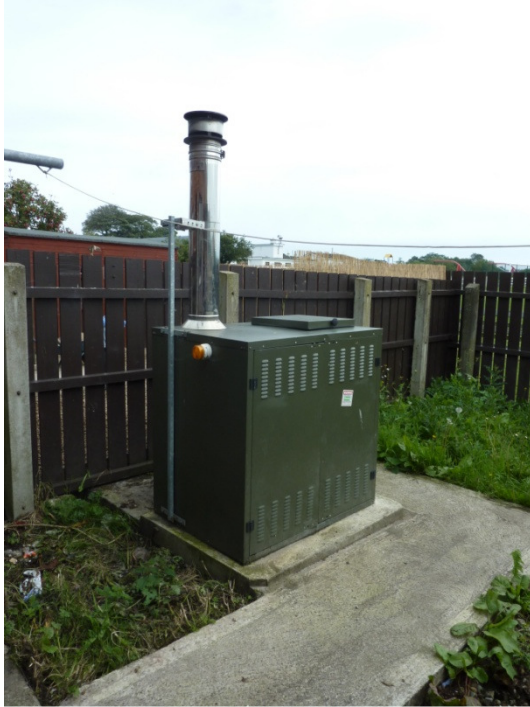
Biomass CHP unit being trialled by NIHE on one of the (as yet) unoccupied properties
