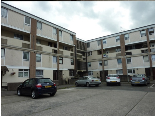
1960s-70s prefabricated flats - would be relatively easy to retrofit due to modular nature of wall panels - can be removed and replaced with similar-sized but insulated panels. These properties often have water ingress issues due to the open balconies. Heat loss thru exposed soffits would be a problem for these as well.
