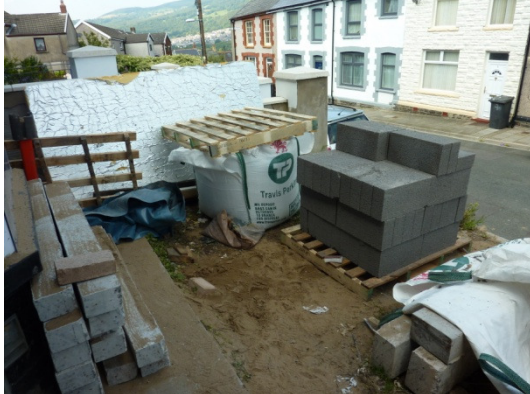
Storage space for construction materials can be a problem on constrained mid-terrace sites. Here, the small front garden is being used for materials storage.
