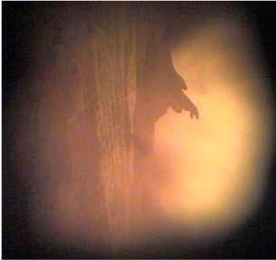
Figure 3.5.11 View from an 'oil burner' video probe prototype, note the slag eyebrow on the adjacent burner.
