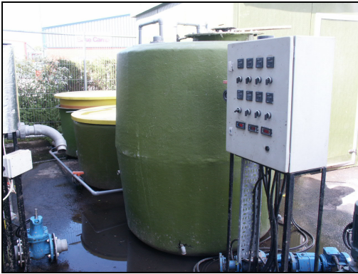
Figure 3. 0.3m 3 Anaerobic Digester
