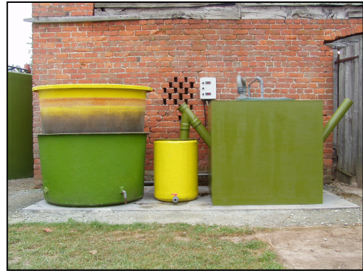
Figure 4. 1.5m 3 Anaerobic Digester
