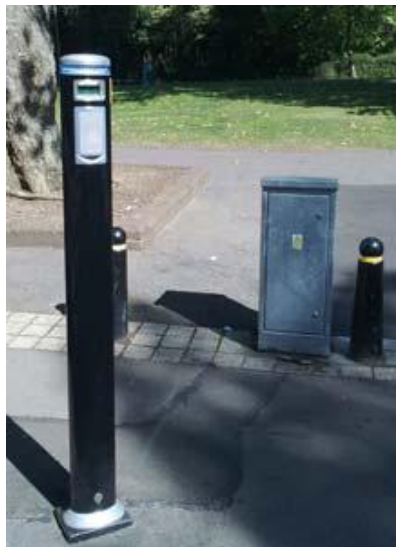
Figure 6: Recharge Post and DNO Owned Feeder Pillar
