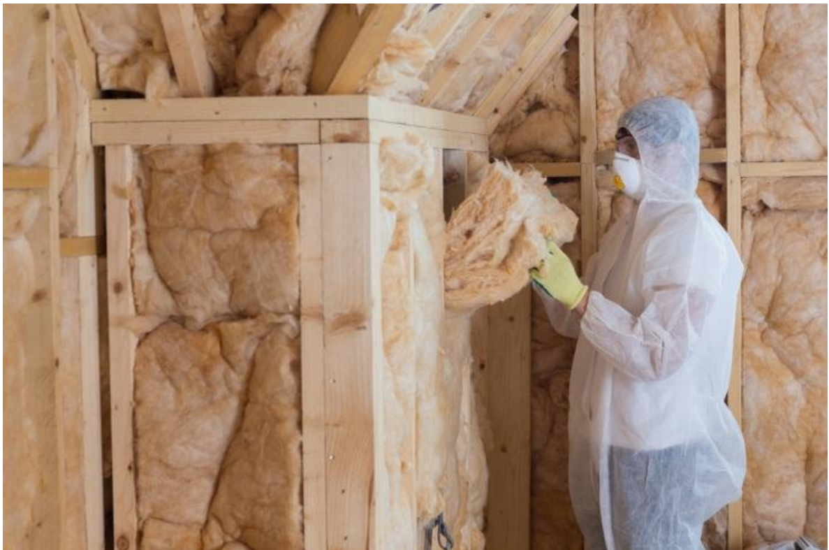
Figure 4.1: Wall and Loft Insulation would not be defined as development and therefore not require planning permission.
