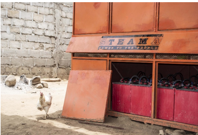
Figure 36: Lead-acid batteries power a mini-grid in Entesopia, Kenya
