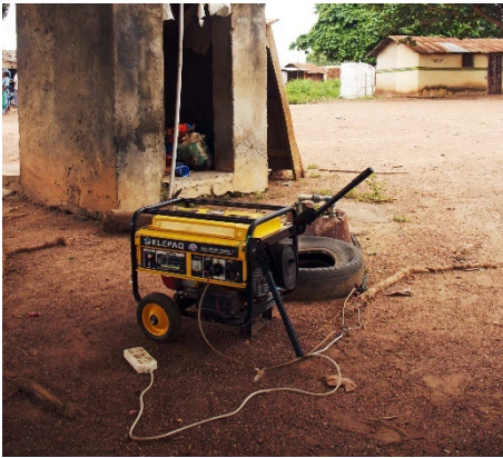
Figure 51: A petrol generator in rural Nigeria runs a water pump
